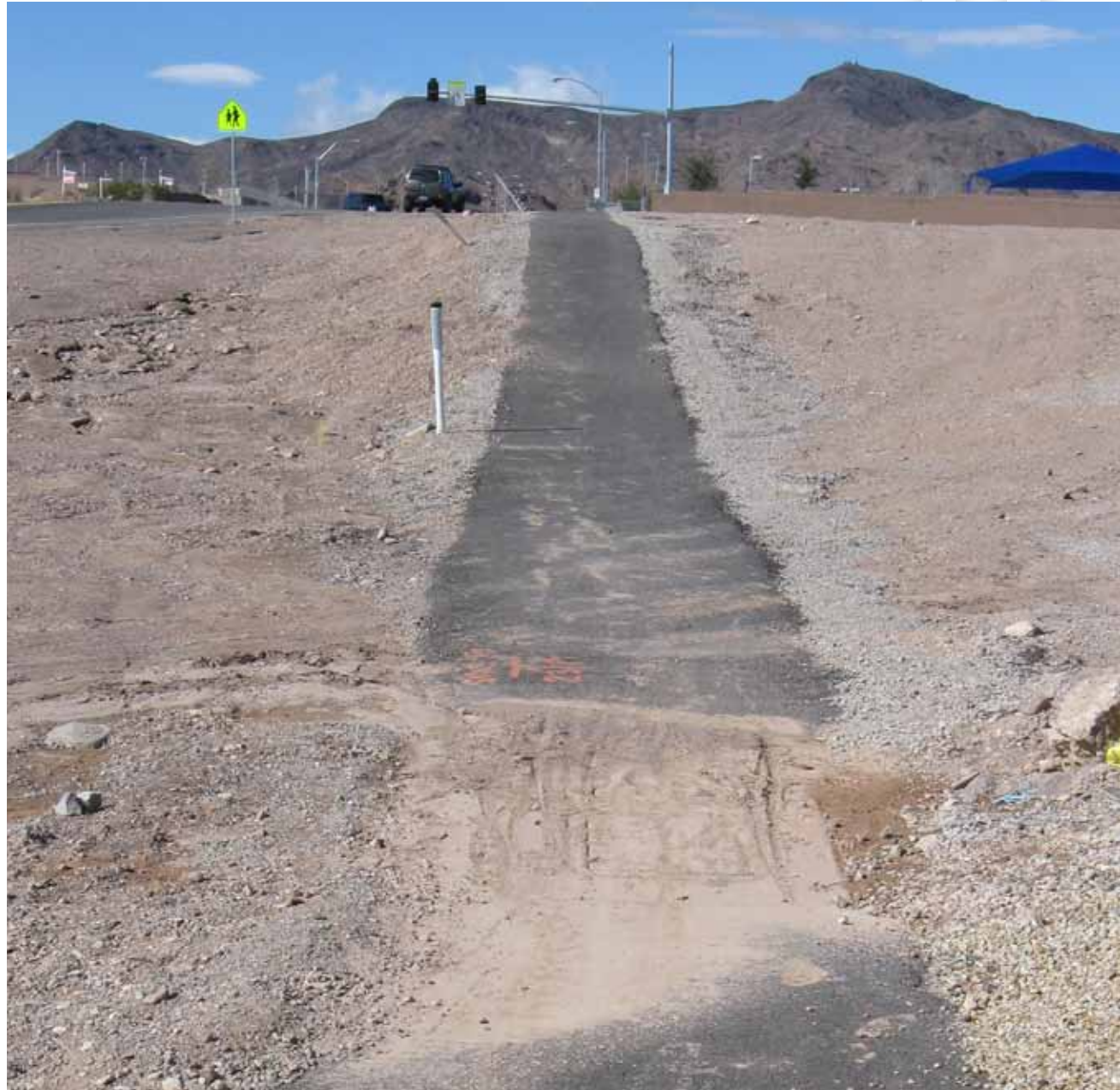
Debris on an asphalt paved trail due to improper drainage design
