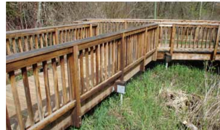
Boardwalk railings assist in keeping trail users away from sensitive areas
